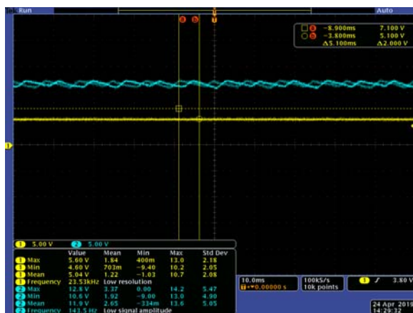
+5 V (yellow signal; max = 5.60 V, min = 4.60 V, mean = 5.04 V) and unregulated 11 V (blue signal; max = 12.8 V, min = 10.6 V, mean = 11.9 V) supplies after repairs.
